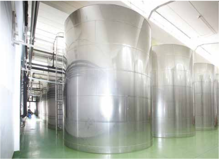
Warehouse B: Insulated Tanks
